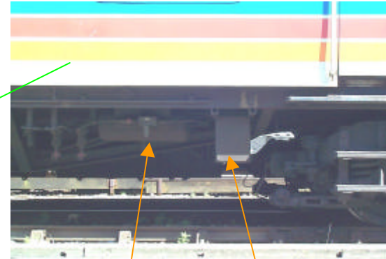
Control air reservoir & Main Auxiliary fuse (Phase 2 only)
