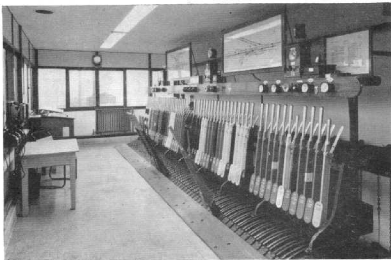
Interior of the new box, showing the lever frame, illuminated diagrams and instruments, with advance indicators set to face the train-booking desk
