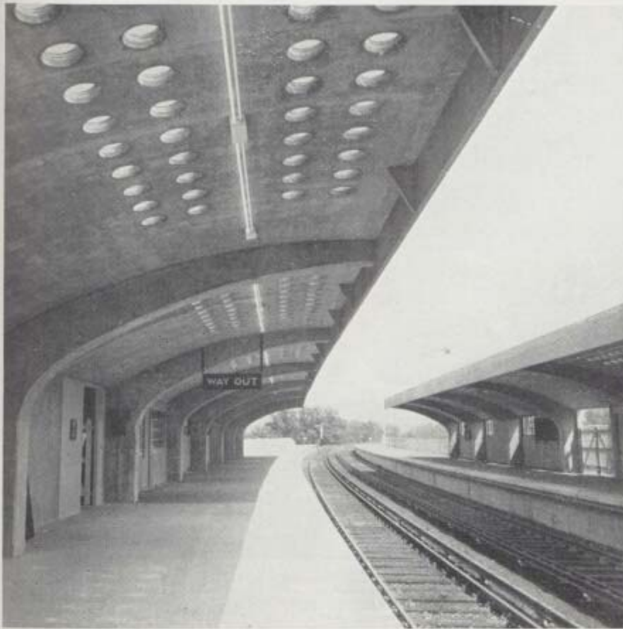
Platforms at Malden Manor station with Chisarc reinforced concrete awnings, free from pillars. Note the fluorescent lighting system
