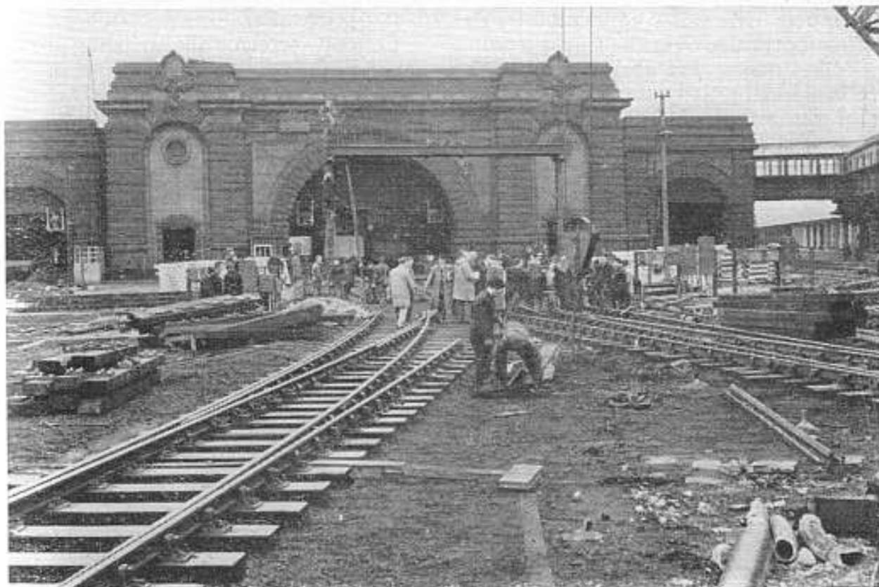
Track alterations in progress at Dover Marine, on the site of platform extensions for electric trains
